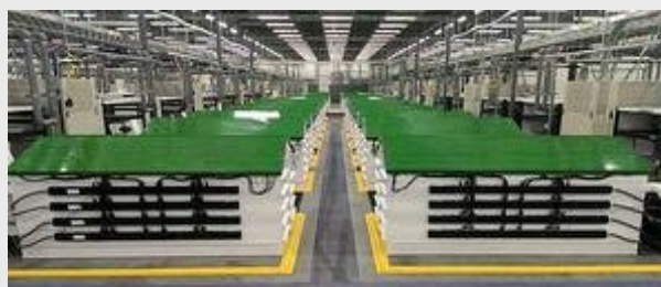
GRC ICEraQ? Immersion-Cooling Installation
